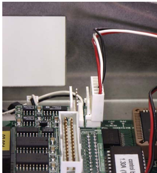
Figure 15 LM35 cable connected to CON1 on TC-board.
